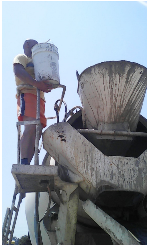
Figure 1. Introduction of the Penetron admix additive in the fresh concrete mass and homogenization of the mixture.
