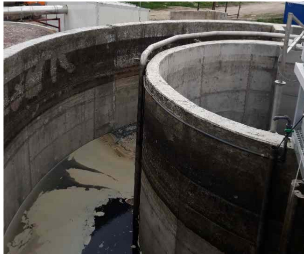
Figure 7. Wastewater treatment station in operation.
