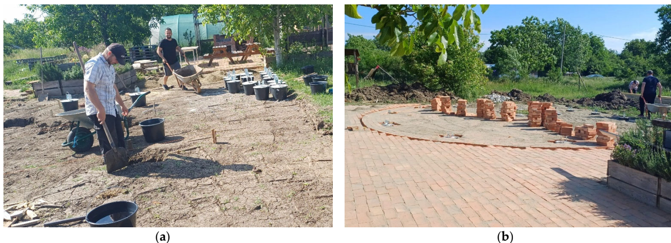
Figure 9. Brick work—recovered brick used for the extension of the existing floor. (a) Preparation of the support for brick layering; (b) brick floor patterning. Images by arch. Amadeea Lazăr.
