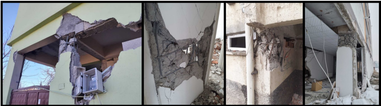
Figure 11. Spalling of core concrete in columns.
