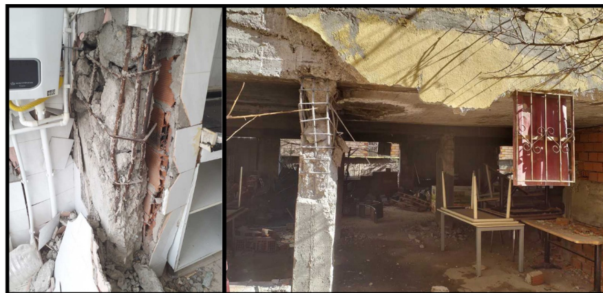
Figure 9. Slippage of reinforcements bent at 90^\circ from the longitudinal reinforcements.
