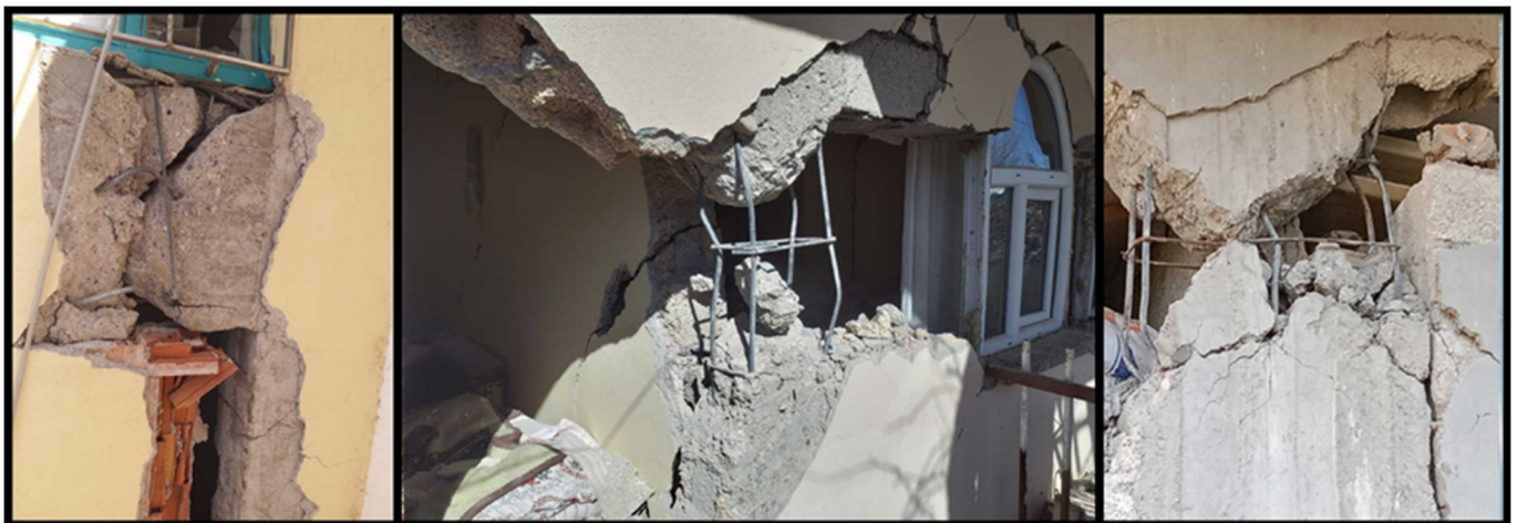
Figure 2. Examples of damage caused by insufficient transverse reinforcement.
