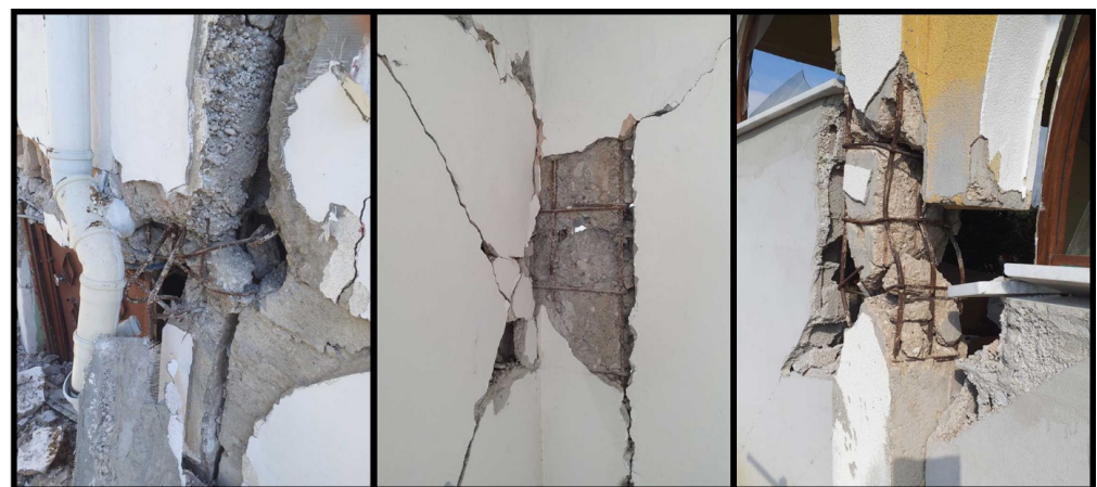
Figure 7. Corroded reinforcement due to insufficient concrete cover thickness and inadequate anchorage.
