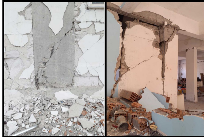
Figure 8. Examples of a shear crack.
