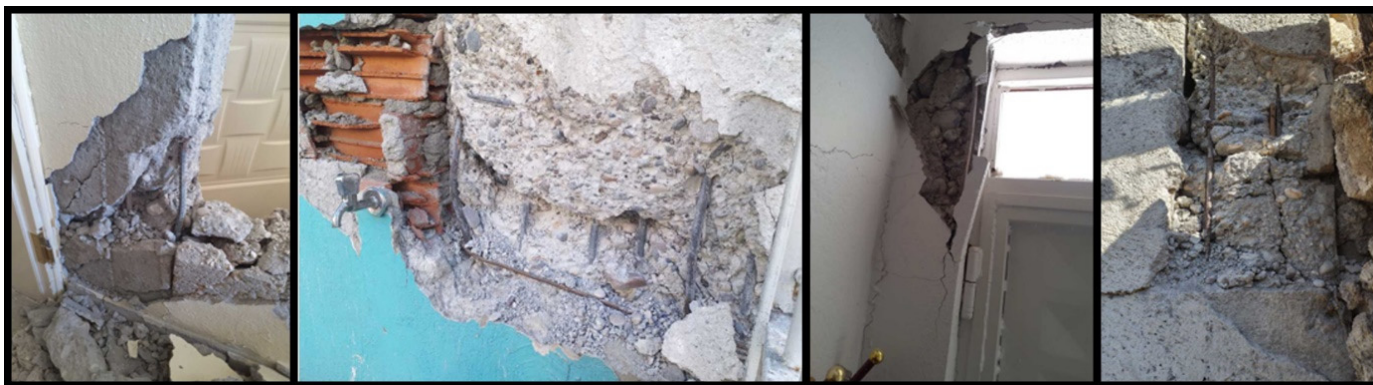
Figure 3. Examples of damage from low-strength concrete.
