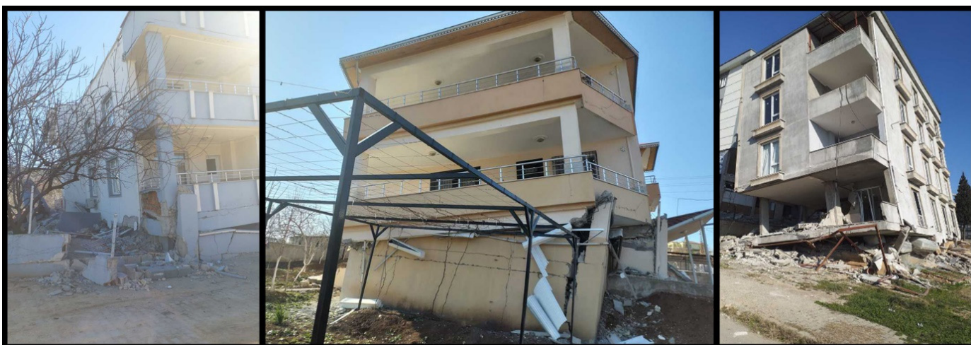
Figure 4. Examples of out-of-plane damage in columns.
