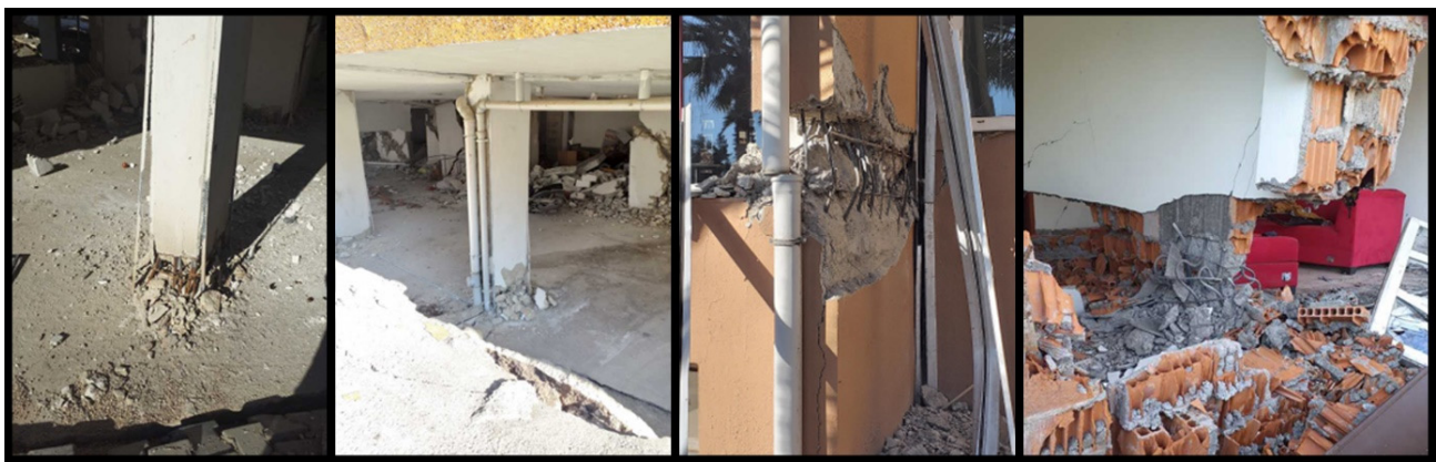
Figure 6. Plastic hinges occur in the lower-end regions of the columns.
