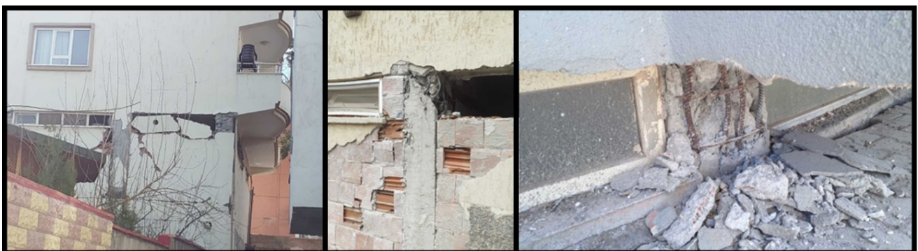
Figure 14. Examples of damage caused by short columns.
