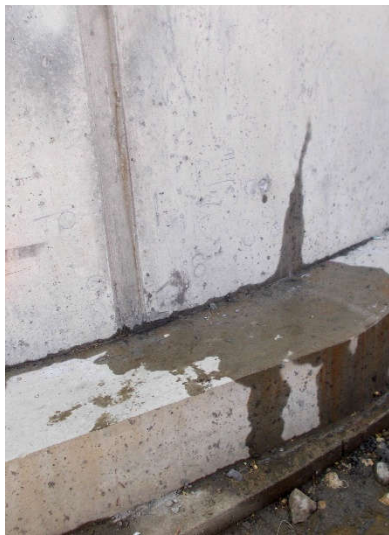
Figure 7. Areas of excessive humidity or leakage at the wall-raft foundation joint.
