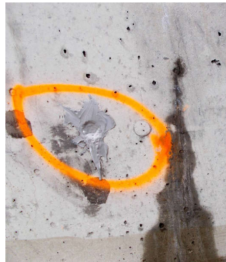
Figure 8. Areas of excessive humidity or leakage on wall.
