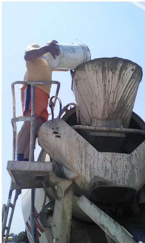
Figure 6. Inserting the Penetron Admix additive into the mass of fresh concrete with at least 15 minutes before pouring.
