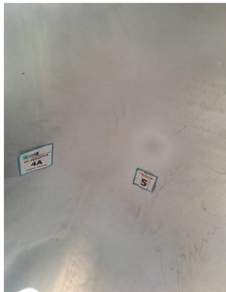
Figure 7. Repaired section of blade no. 5 where the crack was located: back side (top), front side (bottom).
