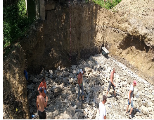
b. Blockage with compacted stone.
