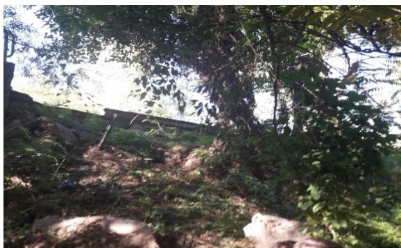
a. Collapsed embankment view
