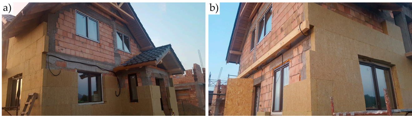
Figure 5. Photographs of the mineral wool insulation of the case study building during the construction stage in 2019: (a) south-east; (b) south-west.
